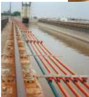
Water Treatment Works
