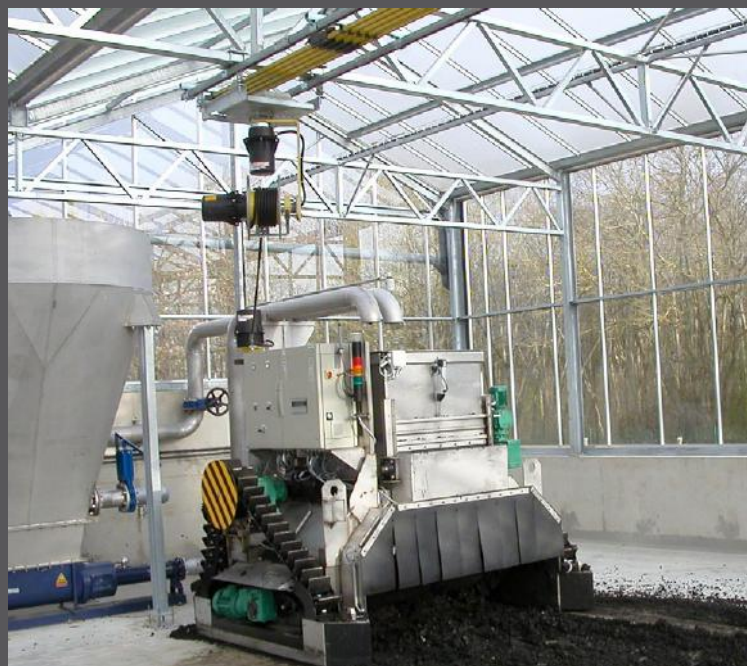
Customized solution with conductor rail, spring reel and slip ring assembly for sludge drying systems
