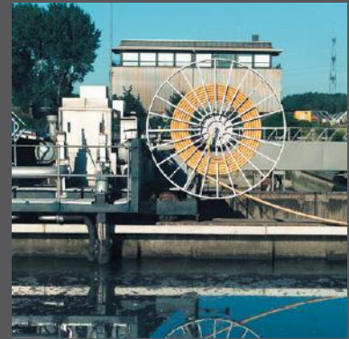
Motorised Cable Reel on a Linear Scraper Bridge
