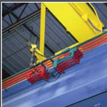
Conductor Bars on an EOT Crane, USA
