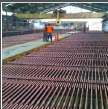
Festoon System on an Electrowinning Process Crane, Peru
