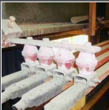
"Dura Coat" Conductor Bar System on an Electrowinning Process Crane, Chile
