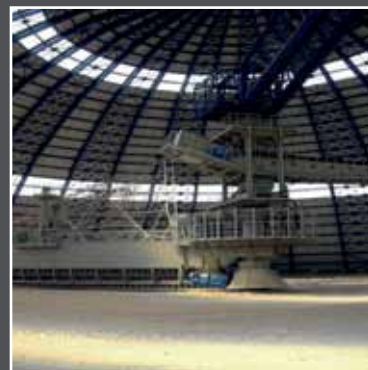
Festoon System on a Circular Bridge Reclaimer, USA
