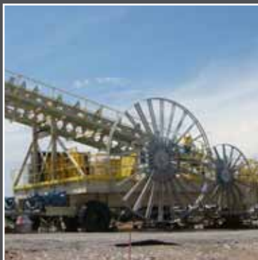
Motor Driven Cable Reels on a Radial Stacker, United Kingdom
