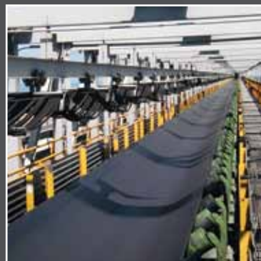
Festoon System on a Tripper Conveyor, Venezuela
