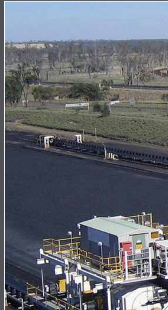
Motor Driven Cable Reel on a Portal Reclaimer, Australia
