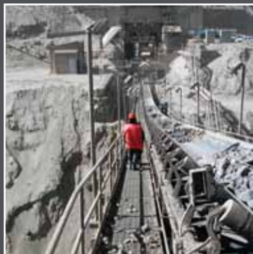
Festoon System on a Conveyor, Chile
