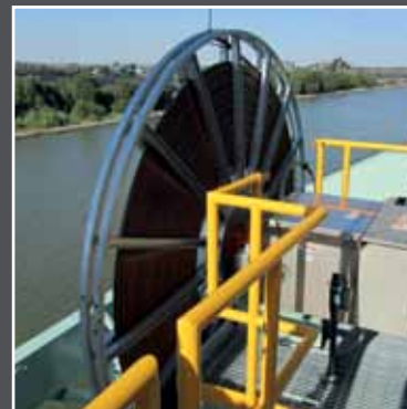
Motor Driven Cable Reels on a Ship Loader, USA
