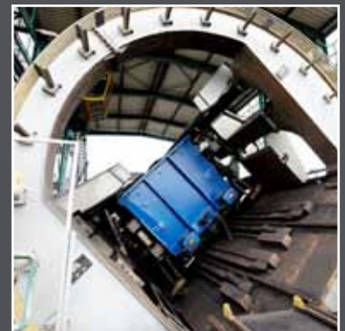
Conductor Bar System on a Rail Car Dumper, Australia
