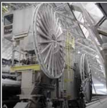
Motor Driven Cable and Hose Reels on a Tripper Conveyor, Venezuela
