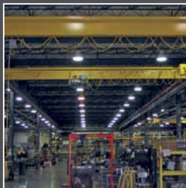
Festoon System on an EOT Crane, USA
