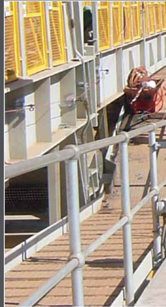
Level Wind Reels on a Stacker/Reclaimer, Australia
