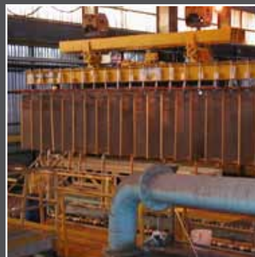
Festoon System on an Electrowinning Process Crane, Chile
