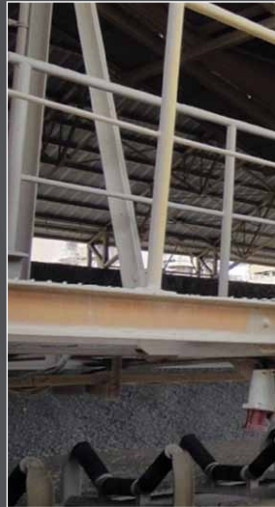
Motor Driven Cable Reels on a Tripper Conveyor, Venezuela
