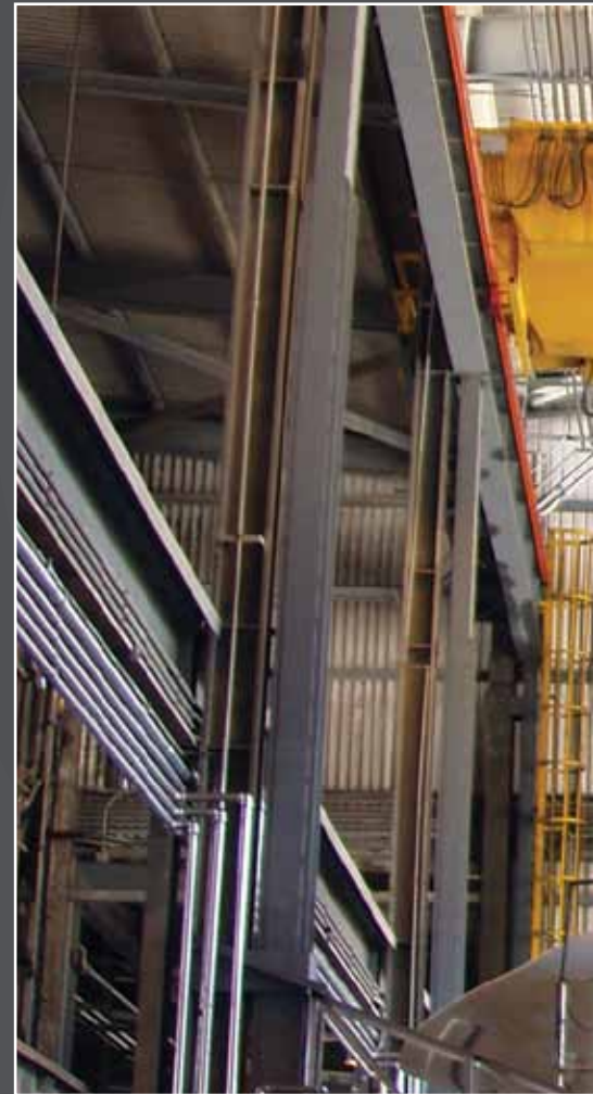
Conductor Bar and Festoon System on an EOT Crane, Colombia
