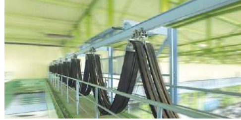
On the go! Cable trolley system program 0350 on a steel mill overhead bridge crane
