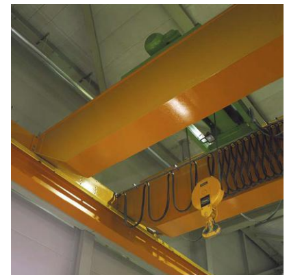
Power supply of the crab on an overhead bridge crane
