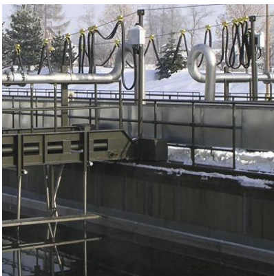
Main power supply of a longitudinal scraper bridge in a waste water treatment plant
