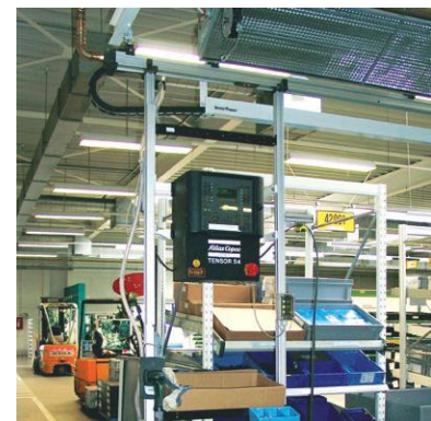
Fully integrated: A62 on an assembly line
