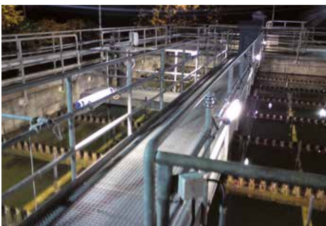
Waterworks street lighting
