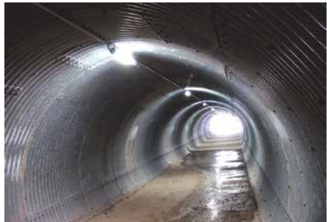
Underpass street lighting
