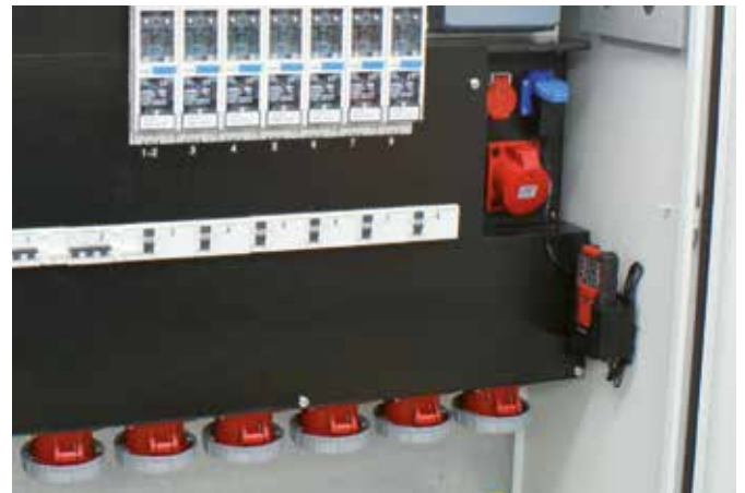
TorchLED torch emergency light in construction site distributor
