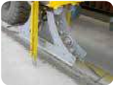
A special “wide” cable guide is used, designed to accommodate lateral movements of the RTG
