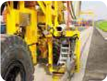
Video cameras monitor the cable trench to assure that the cable remains free to pay out and wind up
