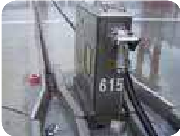
Yard Junction Box with circuit breaker protection, providing the interface to connect the cable reel to the yard power supply
