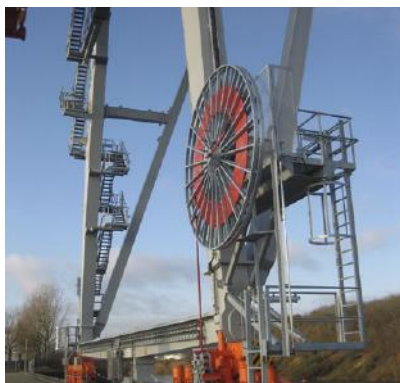
High-voltage main reel cable
