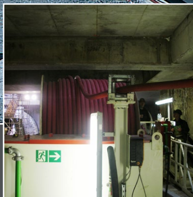
Hydra cable reel feeding power on Tunnel Boring Machine by Herrenknecht
